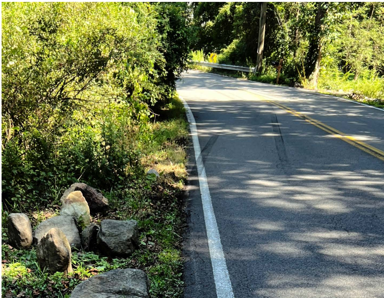
Photo 5 - Accident skid marks and displaced stones 08-22-25
